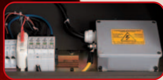
SURGE AND LIGHTNING PROTECTION SYSTEM
